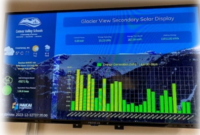
Figure 1 – Glacier View Secondary PV Array Control Panel
