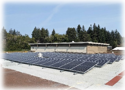
Figure 2 – Glacier View Secondary Rooftop PV Array
