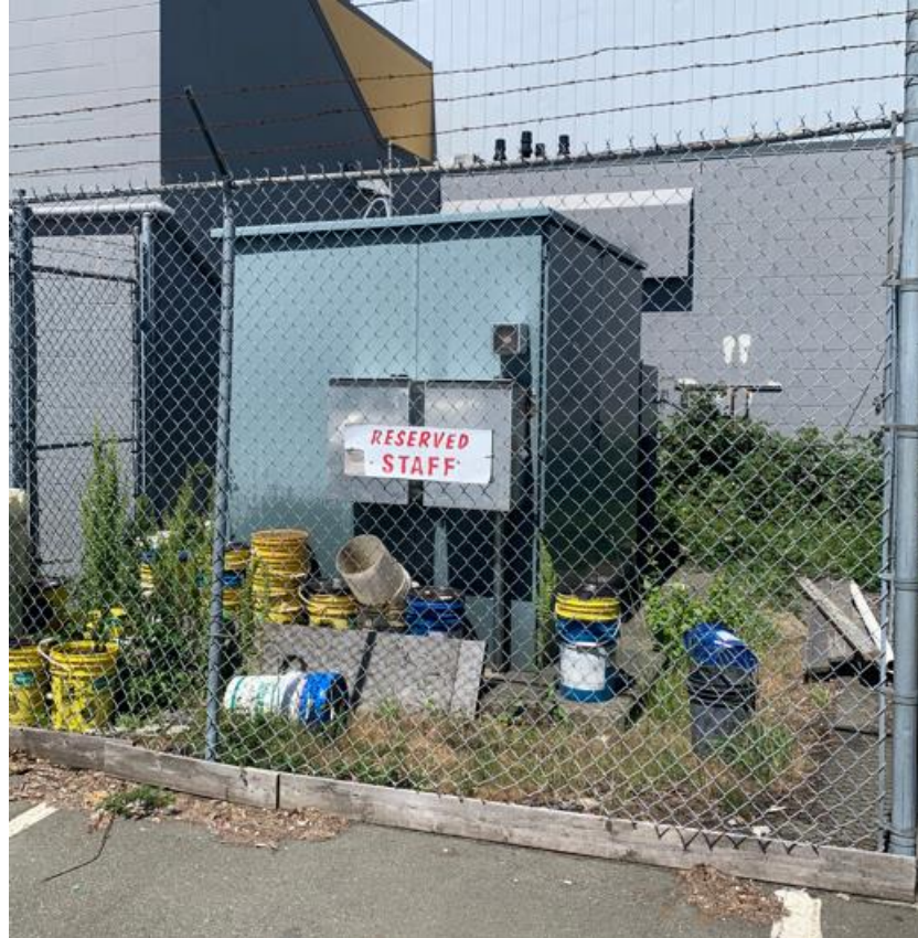
Figure 3: Existing Outdoor Unit Substation
