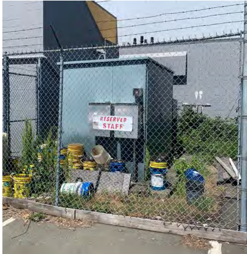
Figure 3: Existing Outdoor Unit Substation
